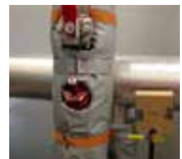
Ganged insulation system
