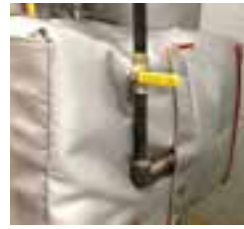
Glycol pump cover
