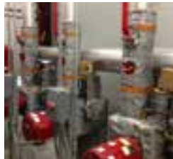
Oil preheat system
